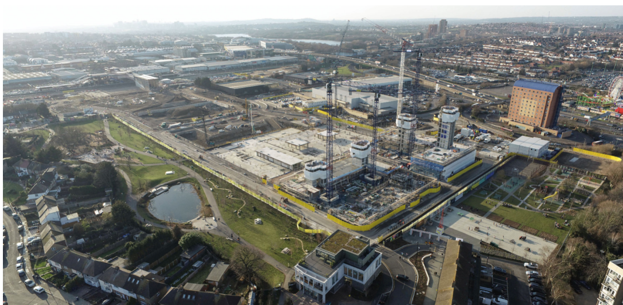
First tower cranes constructed and core of plots 12 and 202 now visible above ground (Feb 23)
